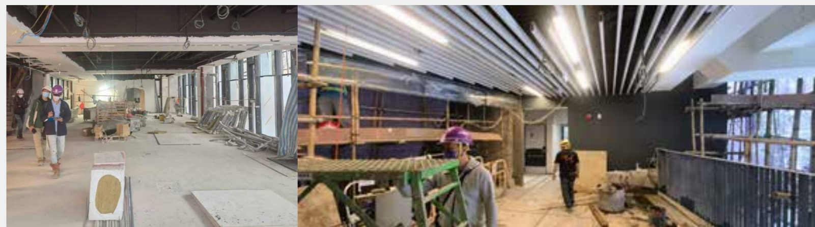
龔約翰學生中心（低座）活動室 Activity Room in “Kunkle Student Centre” (Low Block) 燈光設備安裝 Lighting installation
