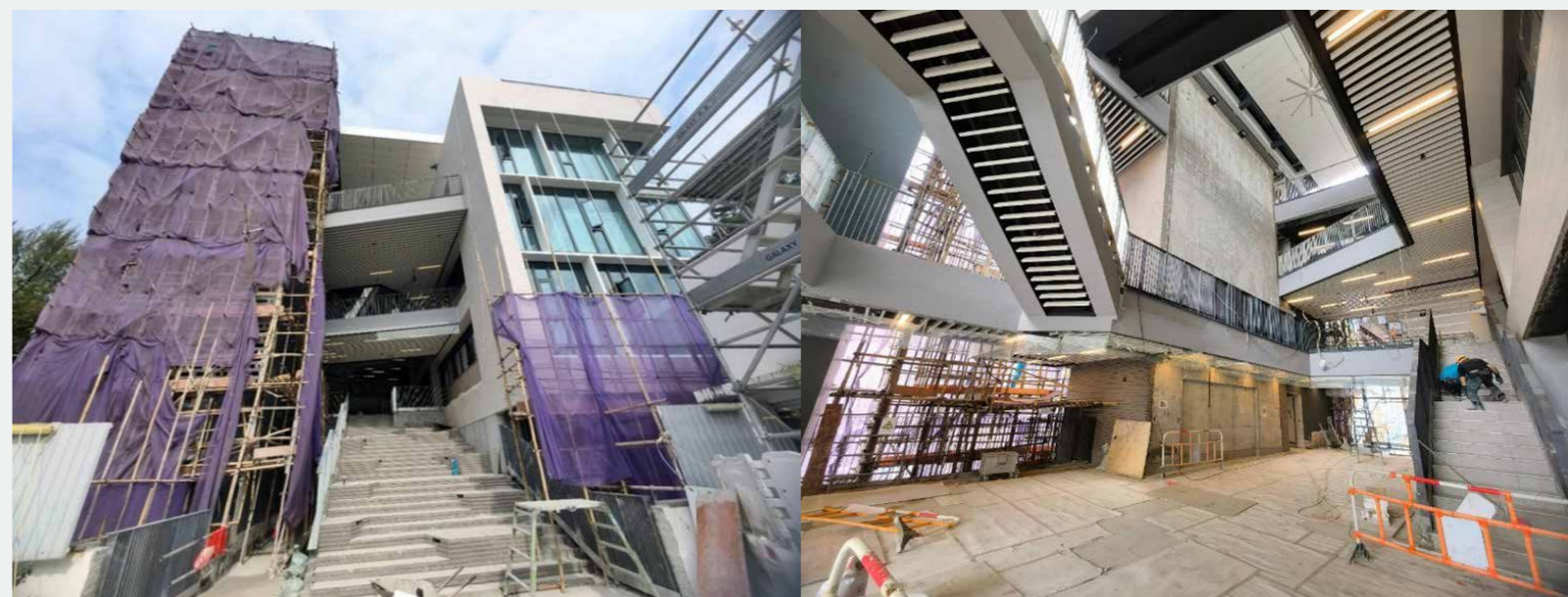
龔約翰學生中心（低座）入口及大堂 Entrance and Lobby of “Kunkle Student Centre” (Low Block)
