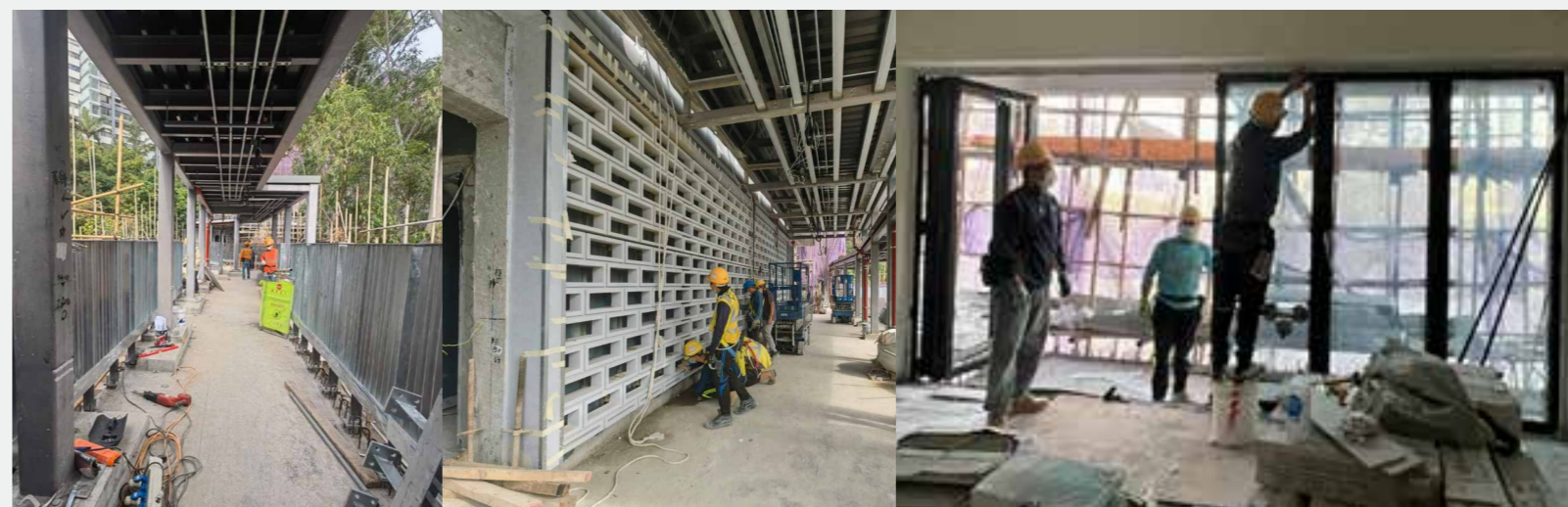
連接高低座的行人天橋 Footbridge connecting High Block and Low Block 梁鳳儀樓（高座）的李福和朱美琳劇院 Fook Wo and Laura Jee Li Theatre in “Leung Fung Yee Building” (High Block) 梁鳳儀樓（高座）教職員宿舍 Staff Quarters in “Leung Fung Yee Building” (High Block)
